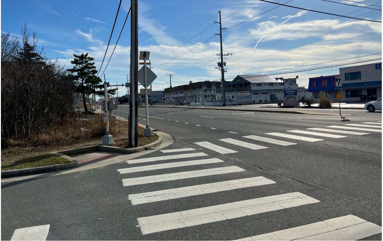
Lack of sidewalks along SR 1 in Fenwick Island
